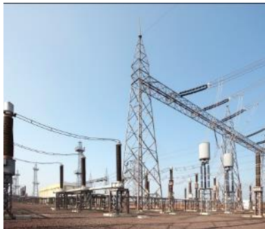
Transmission and distribution
